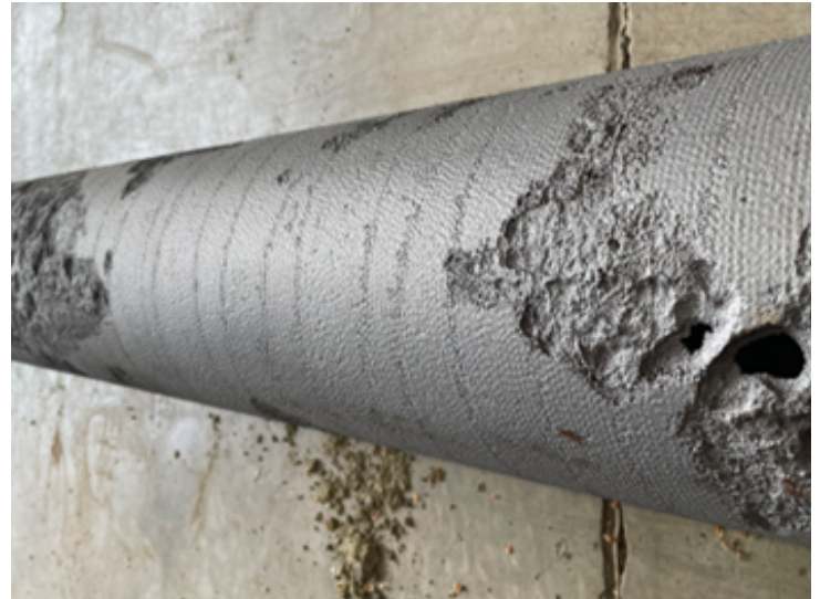
Validation of KenWave DRI technology showing distress on a section of ductile iron pipe.
